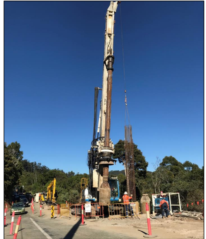
Above: Bored piles under construction near Mirani Street with a steel cage lowered into the ground. Concrete is then pumped into the space around the cage to create the pile.
