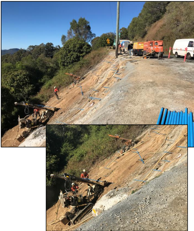
Above: Specialist crews and machinery work on the slip face of this landslip near Bottletree Lane, installing soil nails to stabilise the slope.
